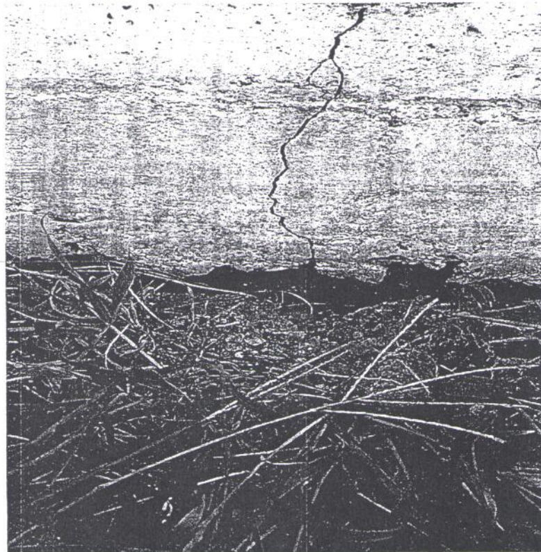
Crack in concrete cap over brick foundation
